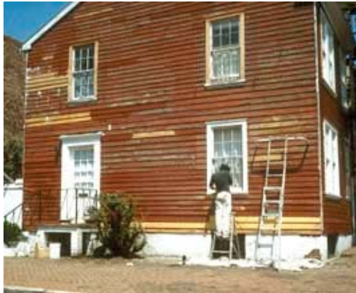
Limited clapboard replacement (Taken from the Secretary of the Interior's Standards for Rehabilitation)
