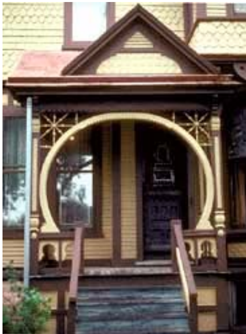
Wood features on porch repaired and preserved during rehabilitation (Taken from the Secretary of the Interior's Standards for Rehabilitation)
