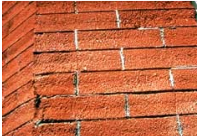
Brick damaged by sandblasting (Taken from the Secretary of the Interior's Standards for Rehabilitation)
